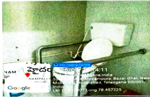
Disabled friendly Washroom.
