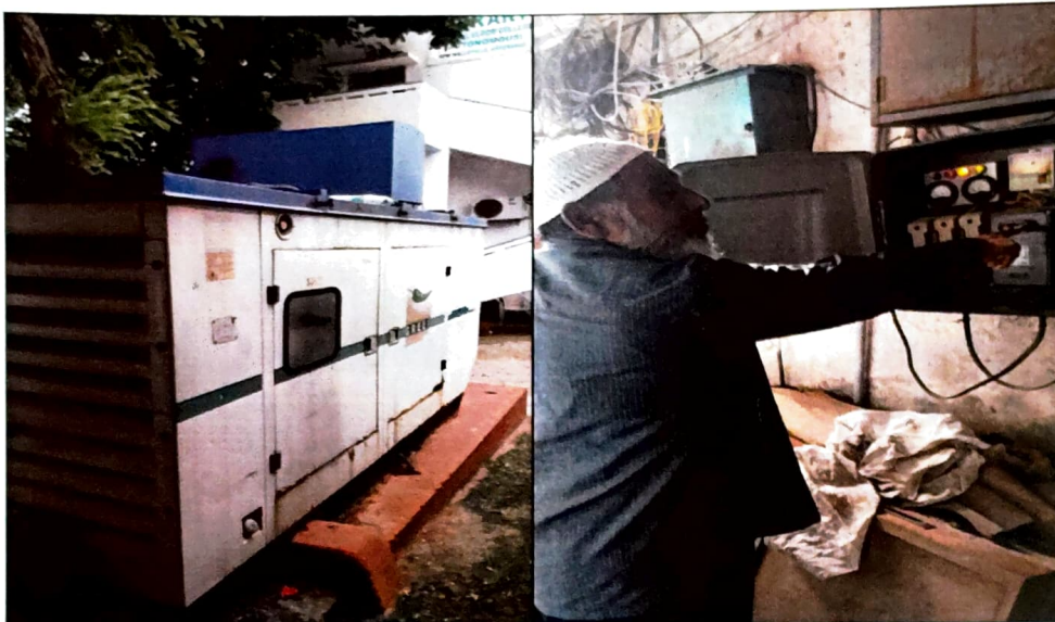
Figure 2.2:- DG set on the college campus
